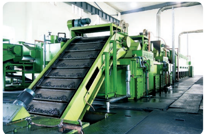
Conveyor furnace line used for roller and bushing heat treatment, e.g. carbon-nitriding
