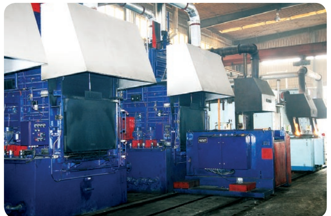
Furnaces for heat treatment process
